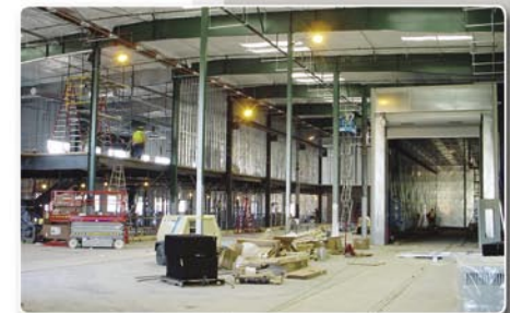
• An expansion of Ruby Junction, (below) TriMet's light rail maintenance shop and storage yard.
